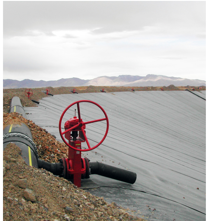
PVM - Series 75 Manual Pinch Valves installed around a mine tailings pond.
