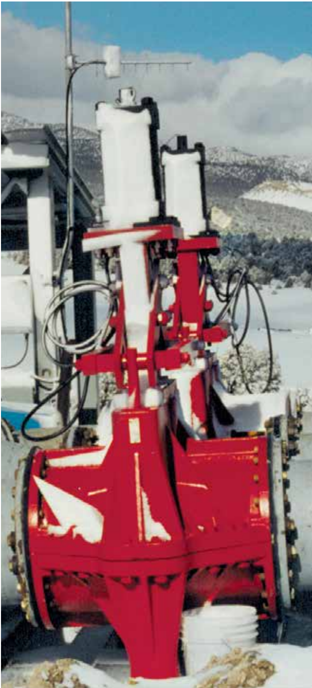
High-Pressure PCV - Series 5400 Pinch Valves on tailings.
